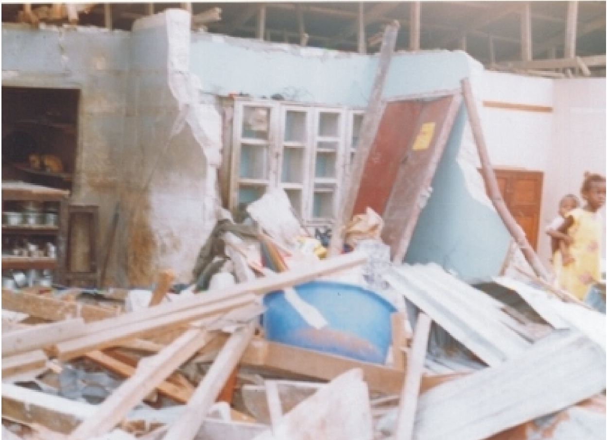
Photographs of some of the demolished residential buildings in Port Harcourt
